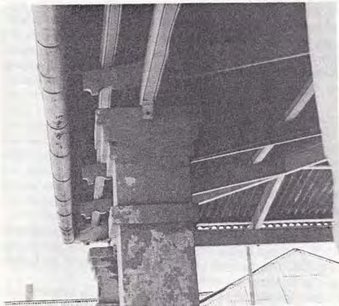
Fig. 25 Directorate of Building Services, Veranda details in the additions to the house of the Deputy Troop Commander, Windhoek, 1902. (Photograph 1979)
